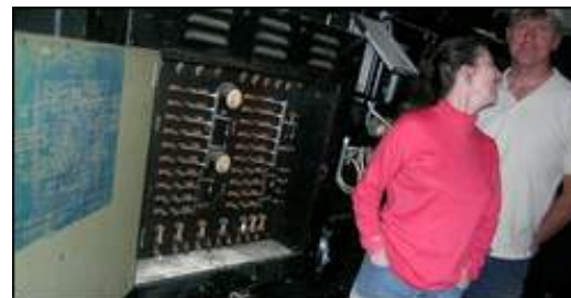
Patricia Splaine looks back at business partner Peter Ejarque as they pass the outdated electrical switchboard that used to power the former Scenic Theater. (Krauss/Democrat photo)
