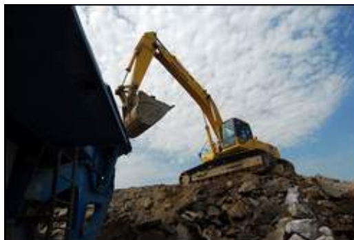
John Huff/Staff photographer Rocky material from The Rochester Shoppes construction site is pulverized into gravel for multiple uses on the location as construction continues along the Spaulding Turnpike in Rochester.
